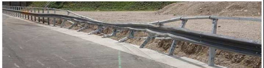
Damage to the device
