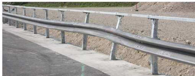
Damage to the device
